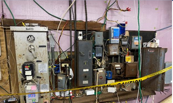
Pump and Well House Interim Emergency Order issued by PA PUC
